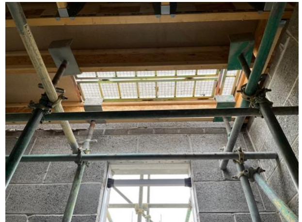
Figure 2. Example of Back Propping that restricts access to the upper floor due to poor planning.
